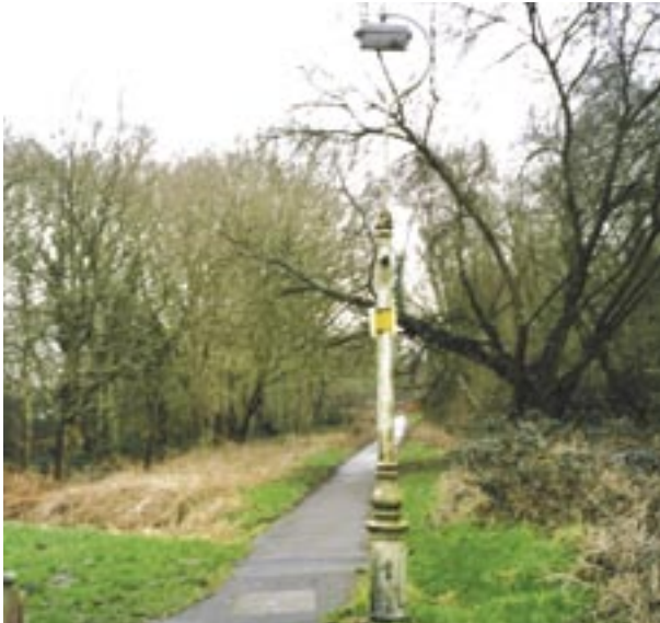
Poorly maintained street lighting
