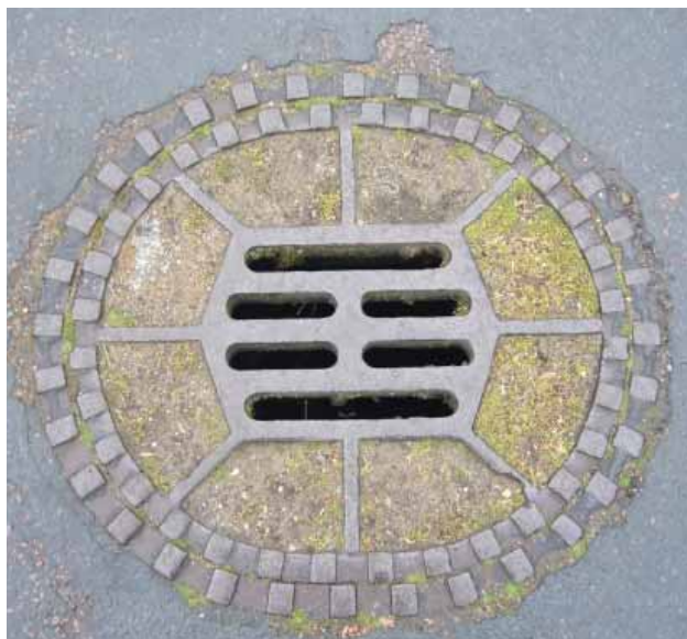
Iron manhole cover
