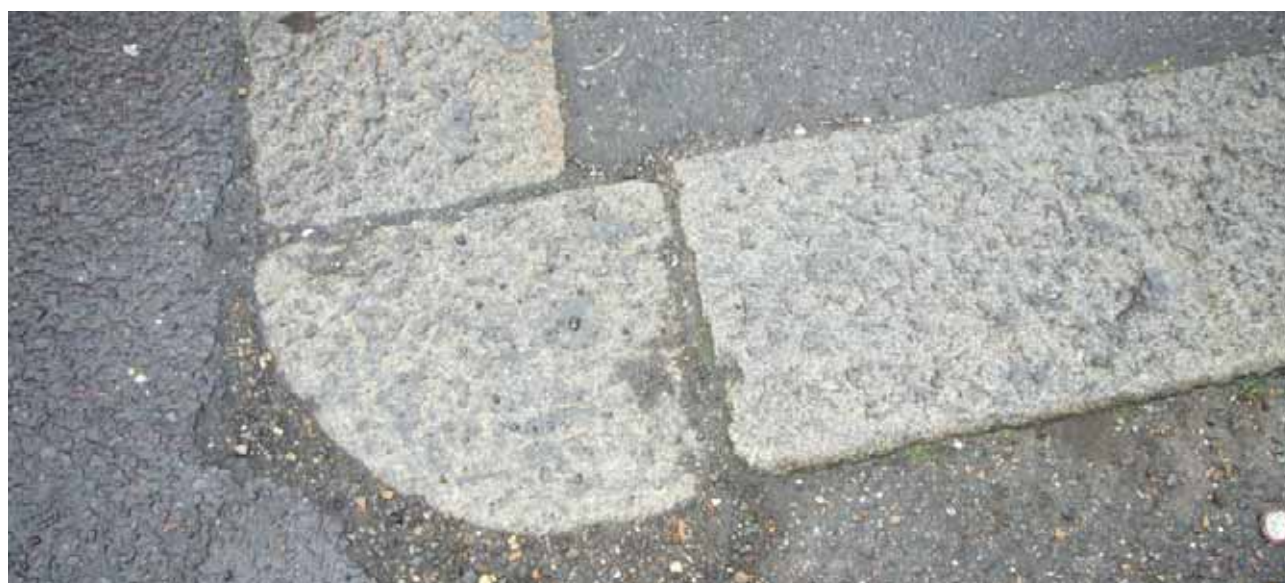
Natural stone kerbs at the junction of Lintons Lane and Middle Lane
