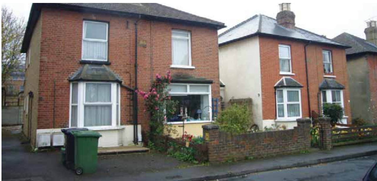
Altered window opening, Victoria Place
