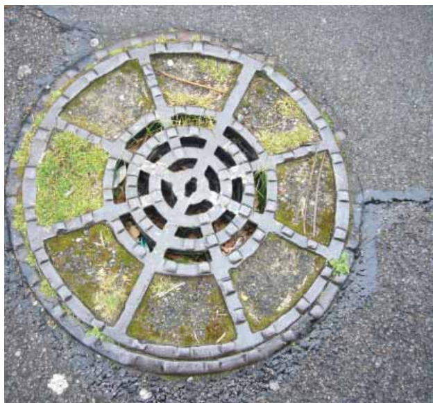
Iron manhole cover
