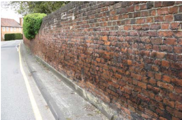
The listed wall in Worple Road to what was once the back garden to The Cedars is in poor condition
