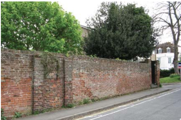
The rear boundary wall to Richmond House faces Downside and is in poor condition
