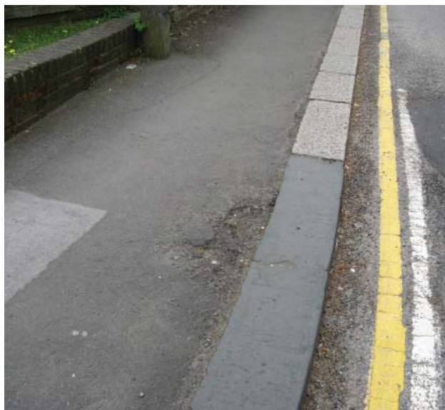
Pavement in Church Street - poor quality surface, but historic stone kerbing has been retained
