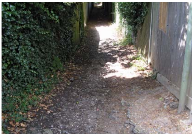
Poor quality paving in the alley off Downs Avenue
