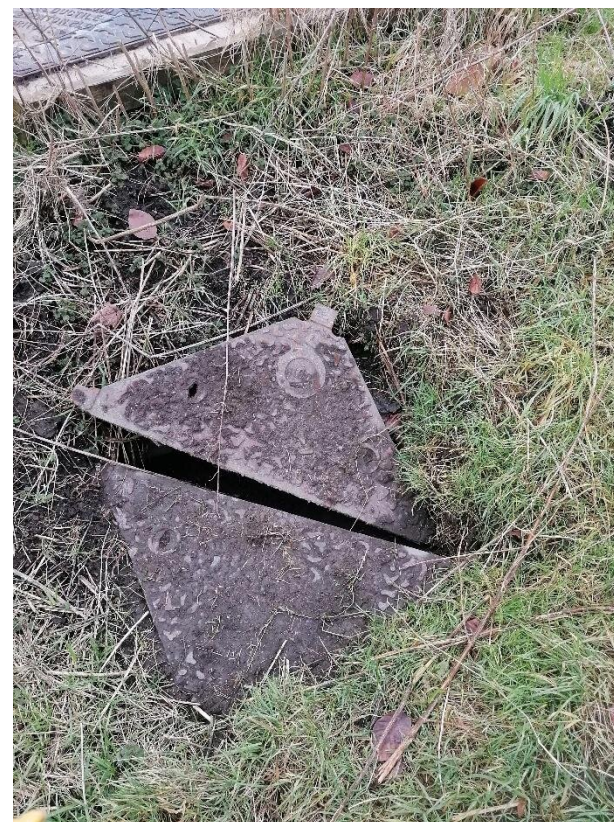
Damaged drain cover at north of Site
