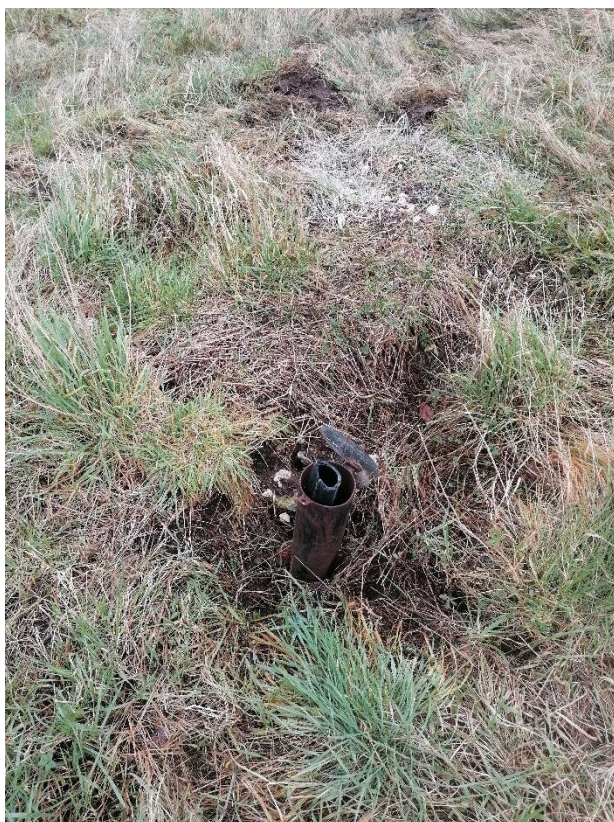
Damage borehole cover at north of Site
