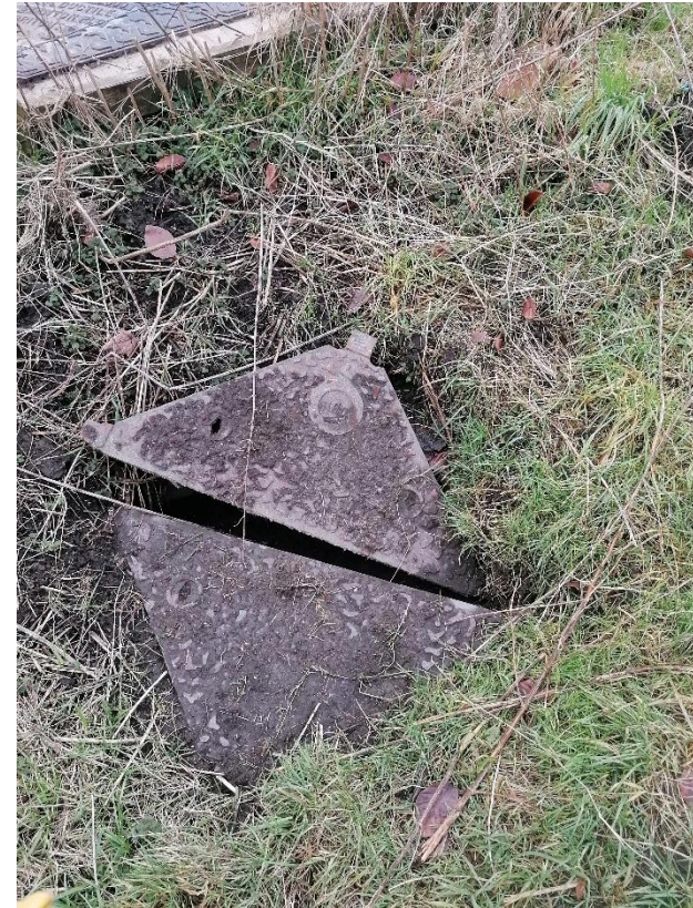
Damaged drain cover at north of Site
