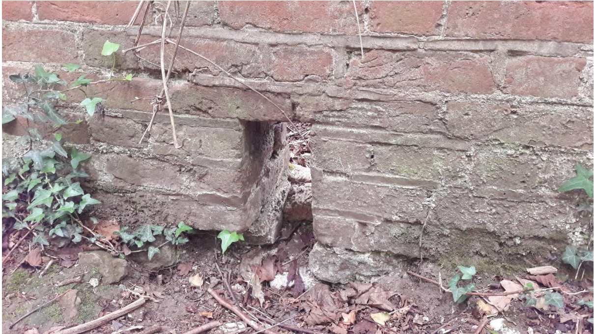
Plate 3: Probable meuse in the south-west wall.
