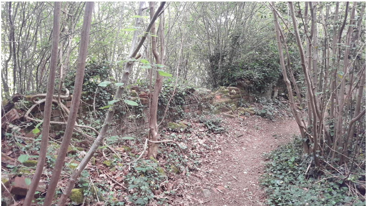
Plate 2: Example of the ruinous condition of parts of the south-west wall, facing west.
