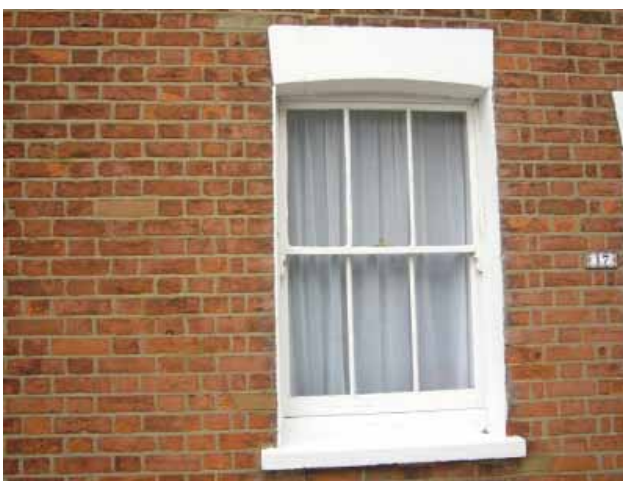
Traditional sash windows in the conservation area need to be protected
